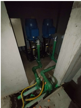
Foto 11 - Instaladas as Bombas de Recalque 15CV
